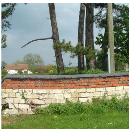
There is little within the village that is "out of keeping" but the wall to the churchyard is in poor condition and parts have collapsed. It is very important that repairs are correctly specified and carefully executed.
